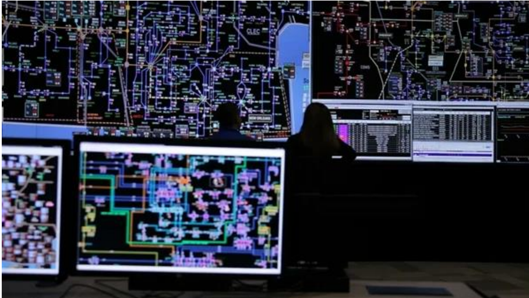
MISO CONTROL ROOM
